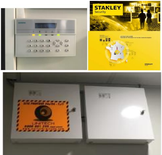
ACCESSE SYSTEM CONTROLLED BY LINTECH
